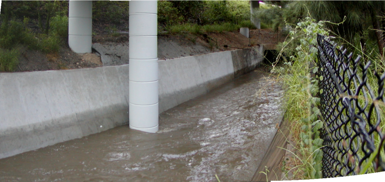
Fig. 6 - Inlet of the Minimum Energy Loss culvert at Marshall Road, Brisbane at the end of a storm on 31 Dec. 2001 - Looking downstream at the inlet flow with one of the concrete piles
